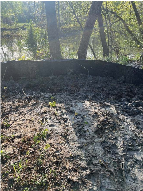
MH 1748 – Sludge against silt fence before cleanup
