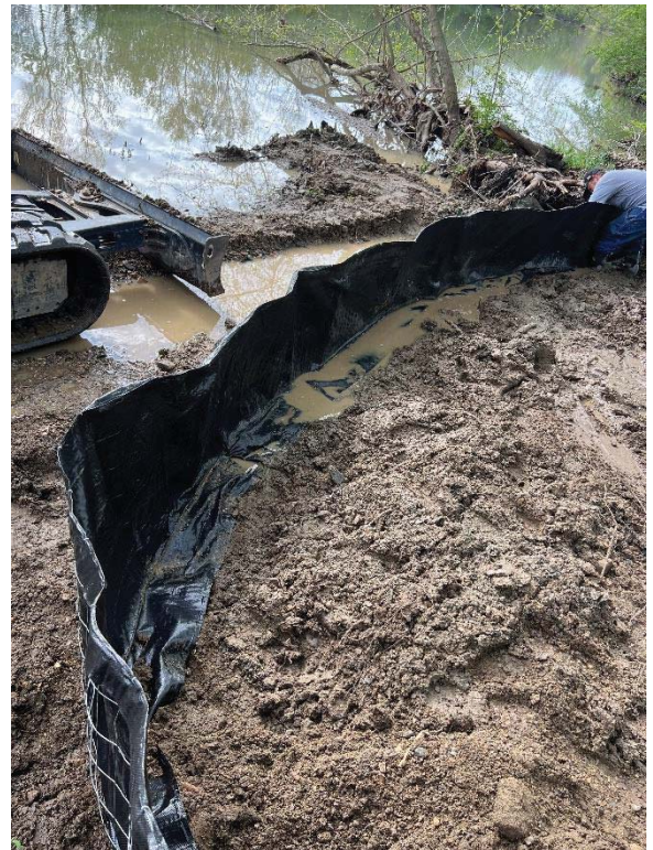
MH 1748 – Sludge against silt fence before cleanup
