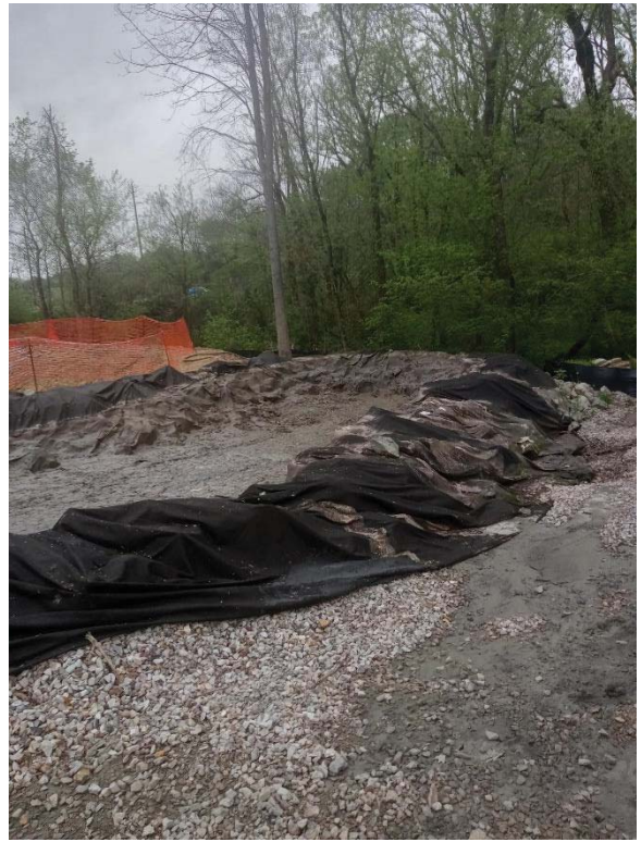
MH 1750 – Sludge in containment berm
