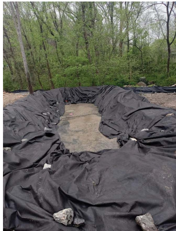
MH 1750 – New liner inside containment berm
